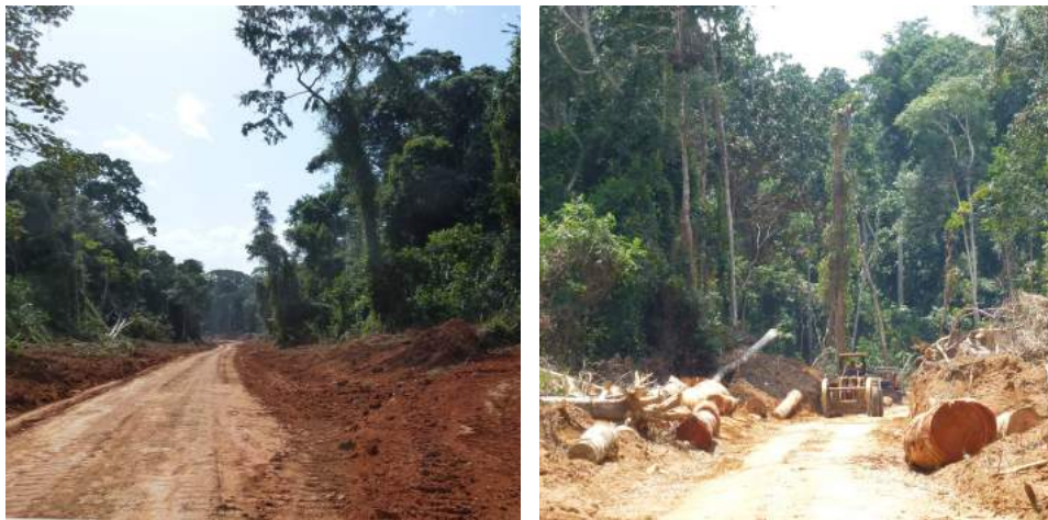
Figure 1.4 – Newly constructed logging roads in south east Cameroon and northern Republic of Congo. Left: Primary road, providing permanent access to the forest. Right: secondary (dead-end) road built for temporary use to collect timber from log landings (here stored on the road side).
