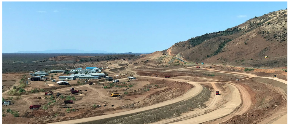
Fig. 2 Construction of an irrigation canal near Omo National Park in southeast Ethiopia (photo by F. Kleinschroth, 29/03/2019)
